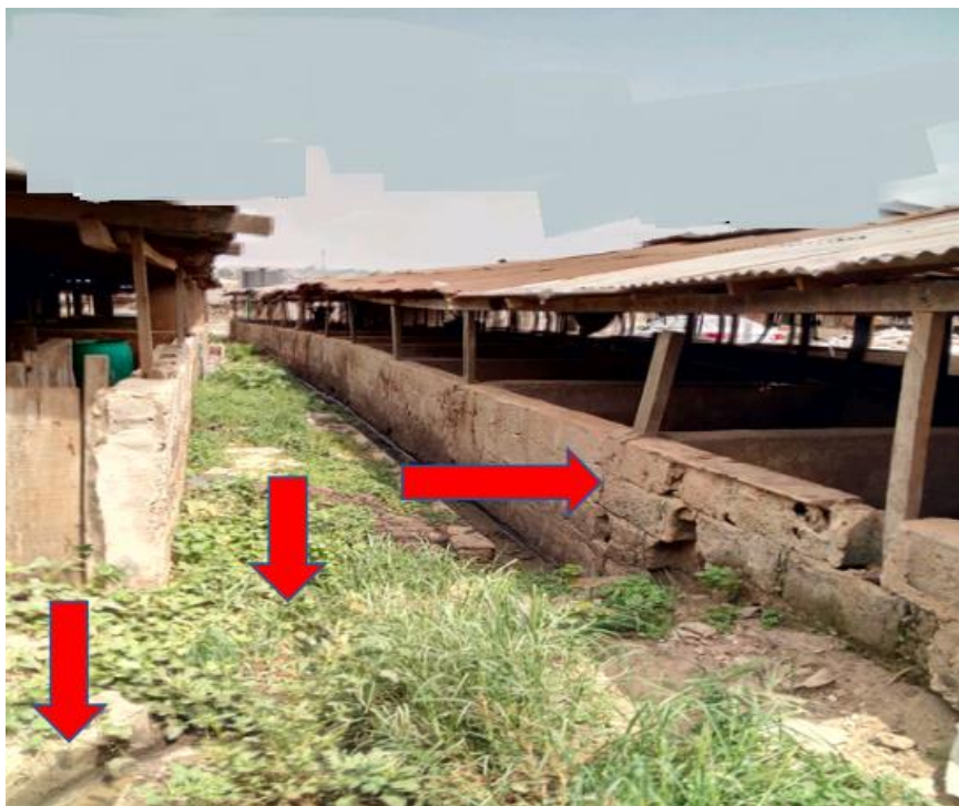
Figure 5: a pig pen with a poor drainage system
